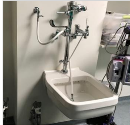
Utility (Service) Sinks
